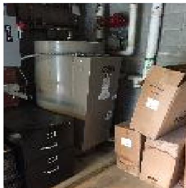
Figure 9 – Domestic Hot Water Equipment
