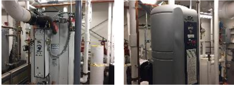
Figure 14 – Domestic Hot Water Equipment
