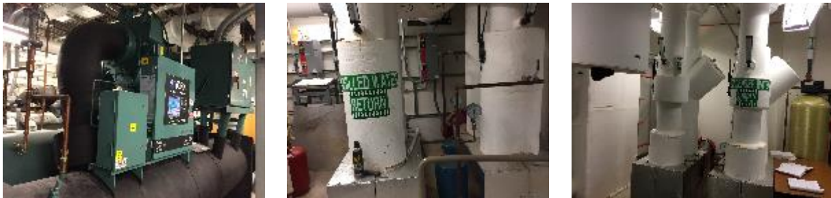
Figure 9 – Chilled Water Equipment
