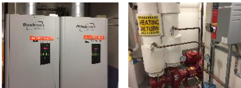
Figure 10 – Hot Water Heating Equipment
