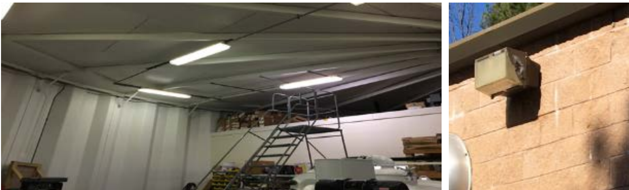
Interior & Exterior Lights
