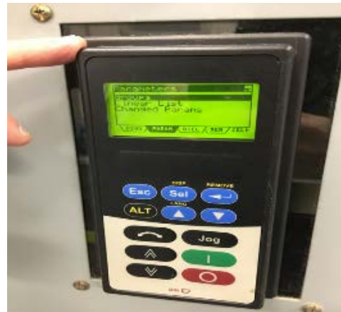
100 hp Well #5 Pump & VFD
