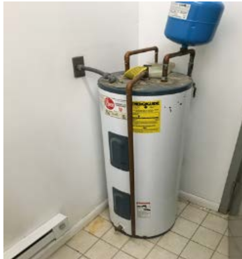
Domestic Water Heater
