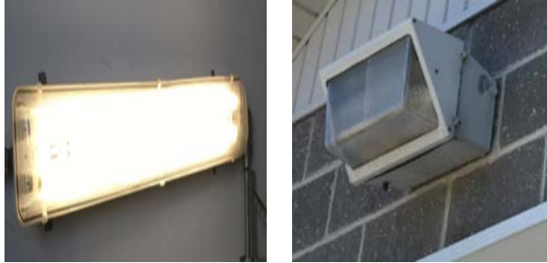
Interior & Exterior Light Fixtures
