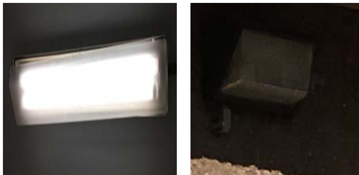
Interior T12 Lamps and Exterior Metal Halide Lamp
