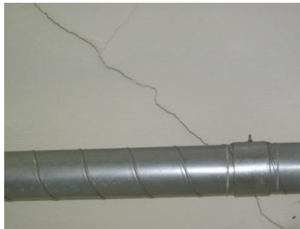
Cracked gypsum wallboard visible in the interior.
