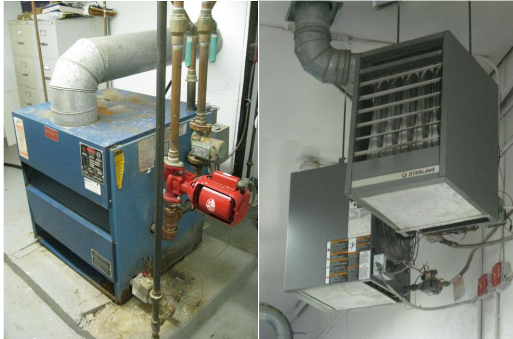
30-year old hot water Utica boiler; ceiling hung gas fired Sterling van / truck bay heaters
