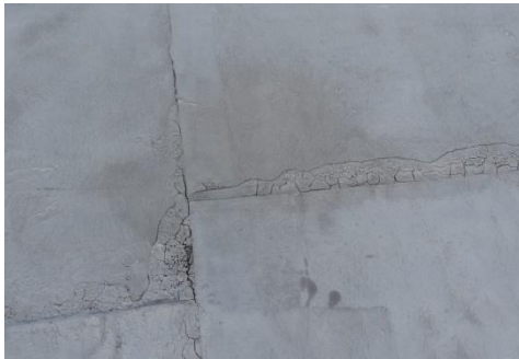
Delaminating / deteriorated roof membrane / patches.
