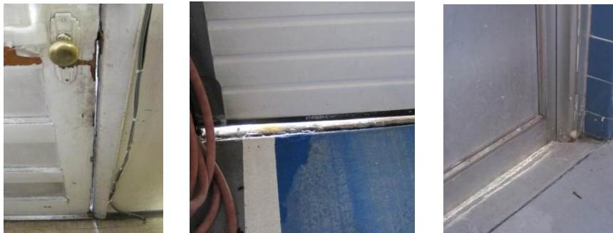
Missing / worn weather stripping at swing and overhead type doors
