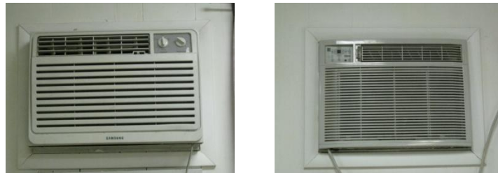
Air-leakage at sleeved window / wall air-conditioning units
