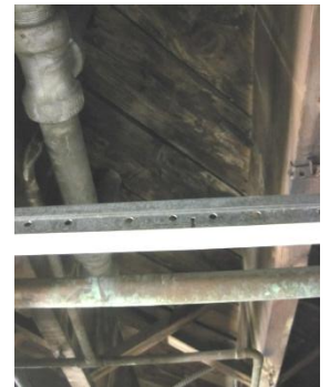
Deteriorating roof decking discovered.
