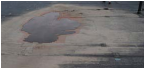
A/C Condensate Water Pooling on Dry Day
