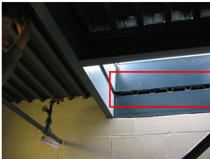
Penetrations found below the roof deck leading to heating/cooling losses
