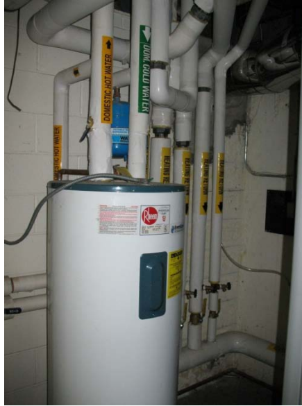
Electric Water Heater
