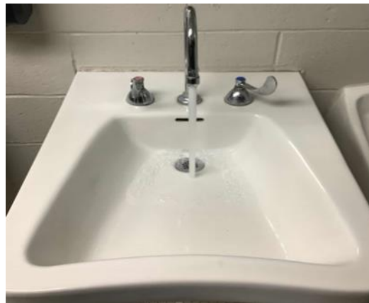
Typical Restroom Sink Flow
