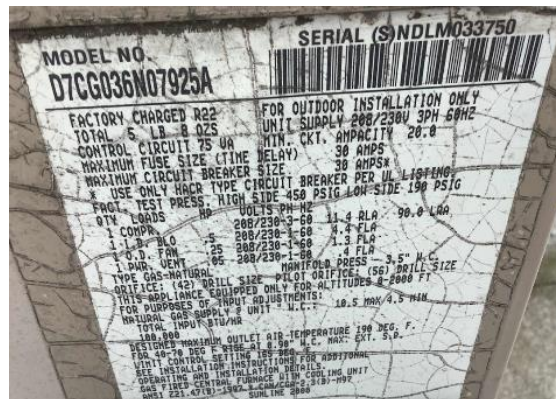
Faculty Room RTU
