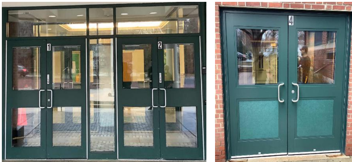
Entrance & Exit Doors
