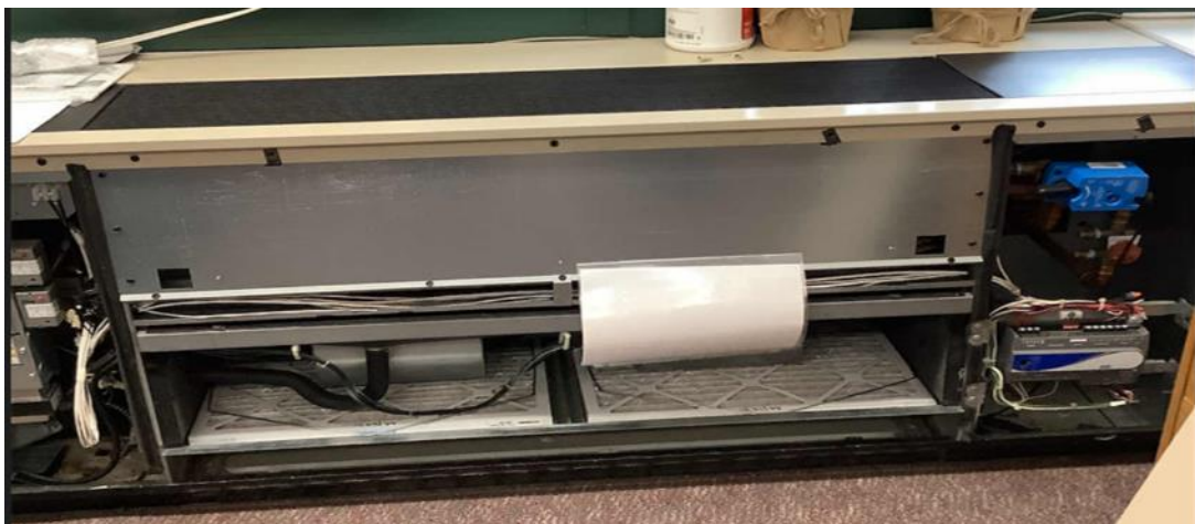
Typical Classrooms Unit Ventilator
