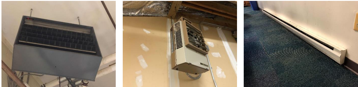
Hot water & electric unit heater, electric resistance baseboard heater
