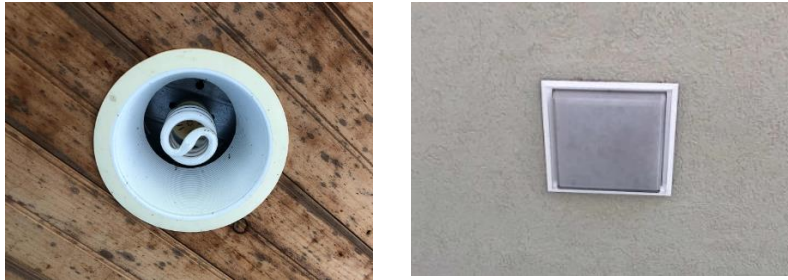
Recessed canopy fixtures
