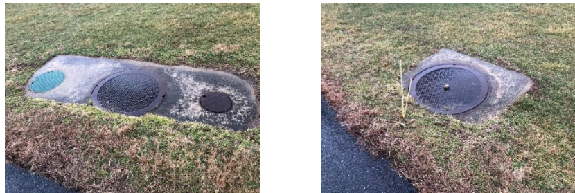
Access hatch for pumps
