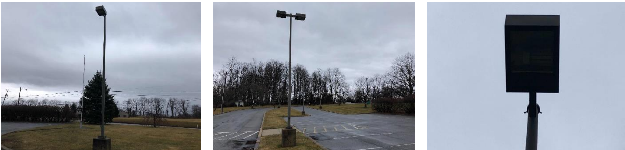
Pole top fixtures
