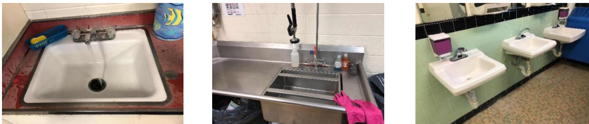
Lavatory sinks and kitchen spray valve
