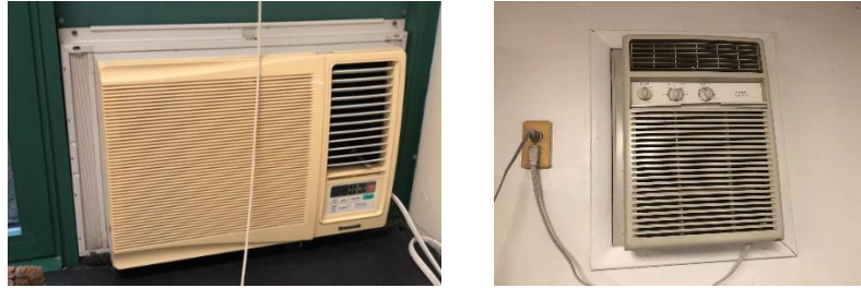
Window AC units
