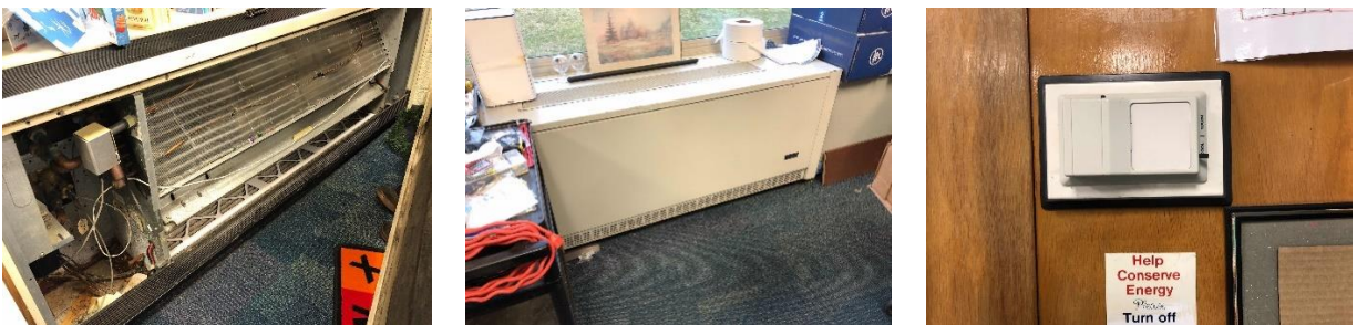
Unit ventilator and thermostat
