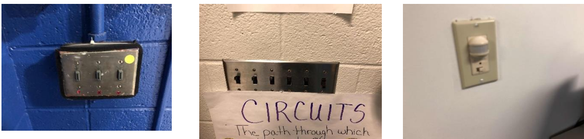
Key and manual switches, and wall switch occupancy sensor
