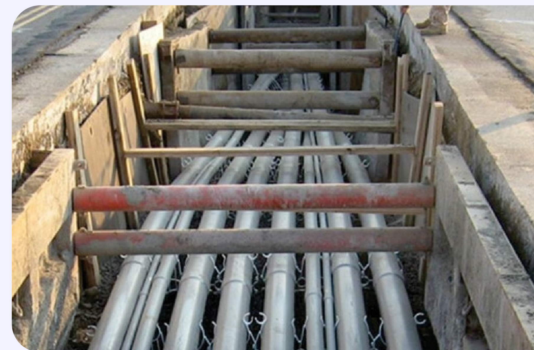
Example of a duct bank
