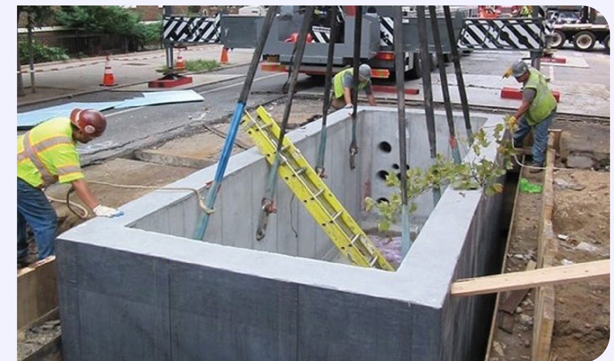
Example of cable vault
